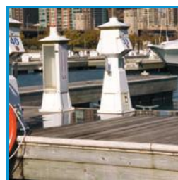
Marine Shore Power & Dock Lighting
