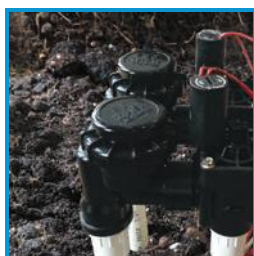
Irrigation & Sprinkler Systems
